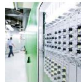
Reparto Building Automation
